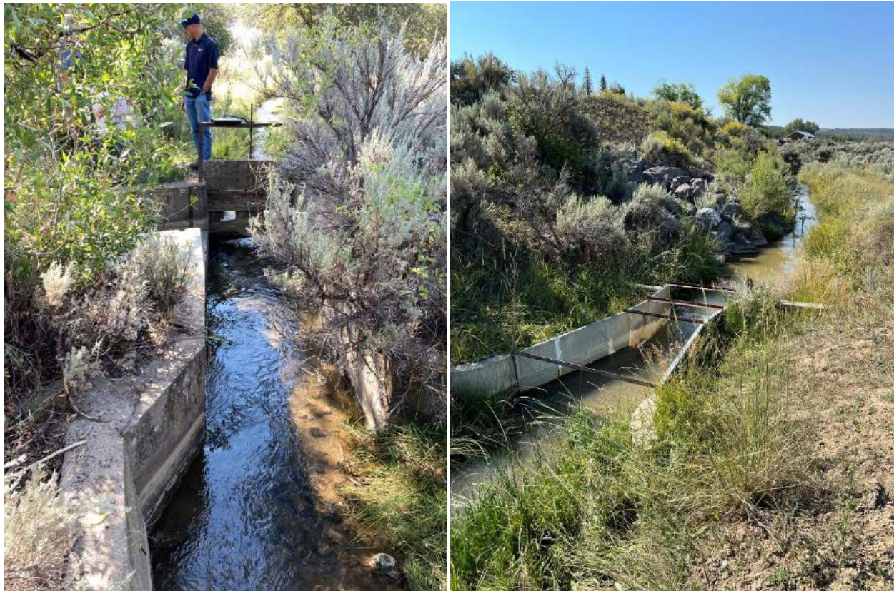
IMAGE 1 & 2: HEADGATE FROM CURRANT CREEK AND 4FT PARSHALL FLUME
